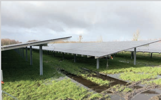
12 MW Barger-Compascuum Solar Park The Netherlands 2018
