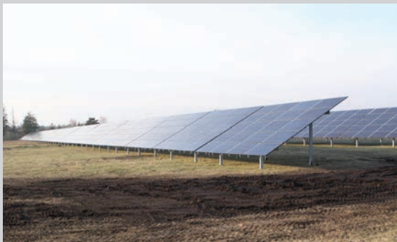
1,3 MW Karup Solar Park Denmark 2016
