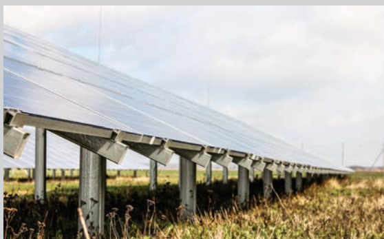
1,1 MW Buczyna Solar Park Poland 2016
