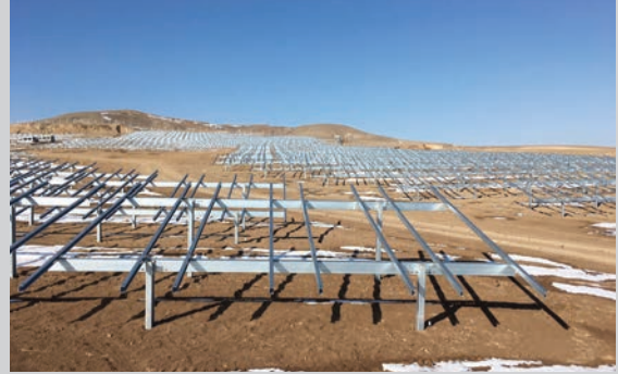
6,1 MW Elaziğ Solar Park Turkey 2017
